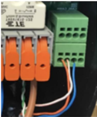
Good installation of meter connections (note RXTX and bridge)
